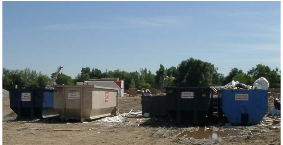
Photo credit: Boulder Associates Architects, 2003. On-site roll-off dumpsters are used to separate and collect construction demolition and debris.
